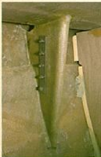
Oversized stainless steel chain plates with backing plates
